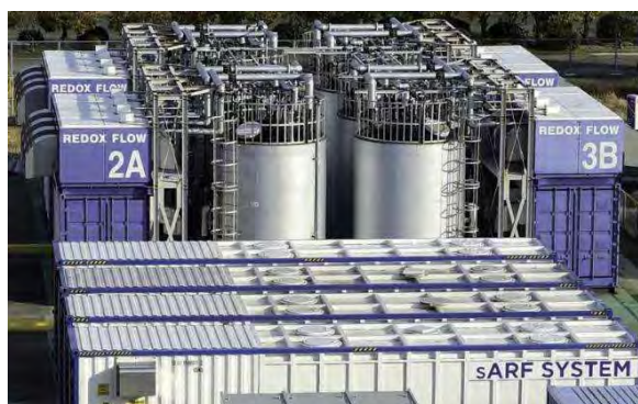
Figure 4: A flow battery installation by Sumitomo Batteries | Sumitomo Electric Industries
